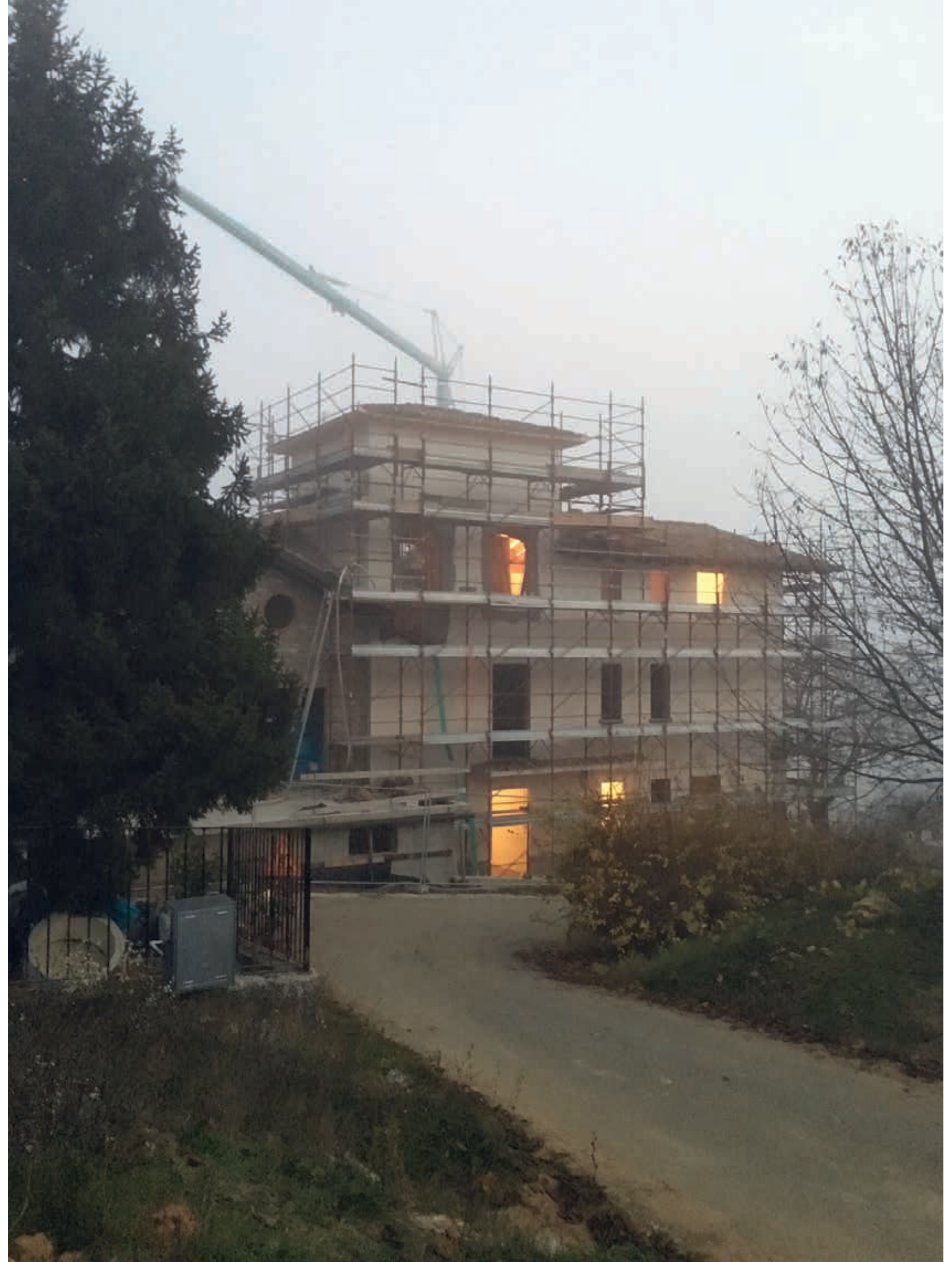
FRANCISCO CORTINA AND ROBERT KILL, architect friends of Marie and Annica, have played a crucial role in the renovations of Villa La Madonna.
